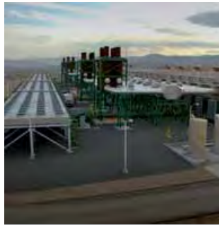
Grid stability and peaking
